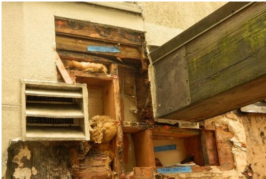
The Fix Building Water Damage
