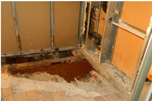
Rose Hill Plaza Water Damage
